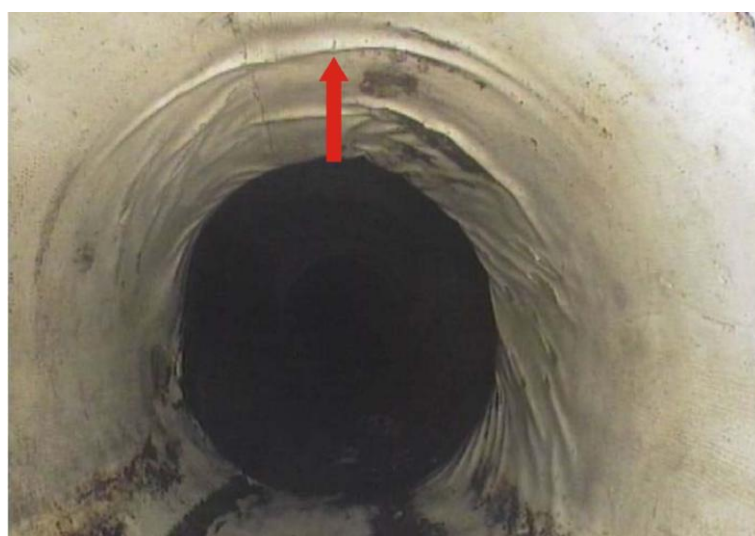
Figure F.28 — Example of lining defect (defective reopening of connection)
