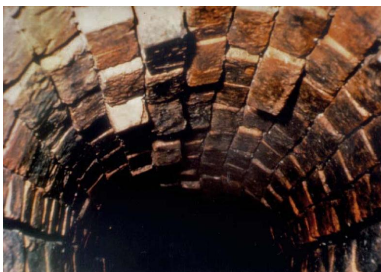
Figure F.12 — Example of collapse
